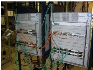
Datacom: Enterprise Switch
