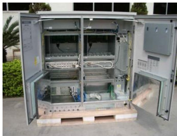
Telecom Wireless Base Station
