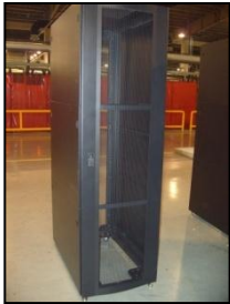
Datacenter Server Rack
